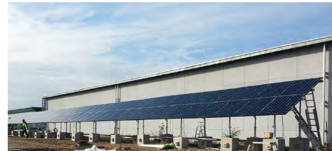
Solar panels at the Bodleian Libraries Book Story Facility
