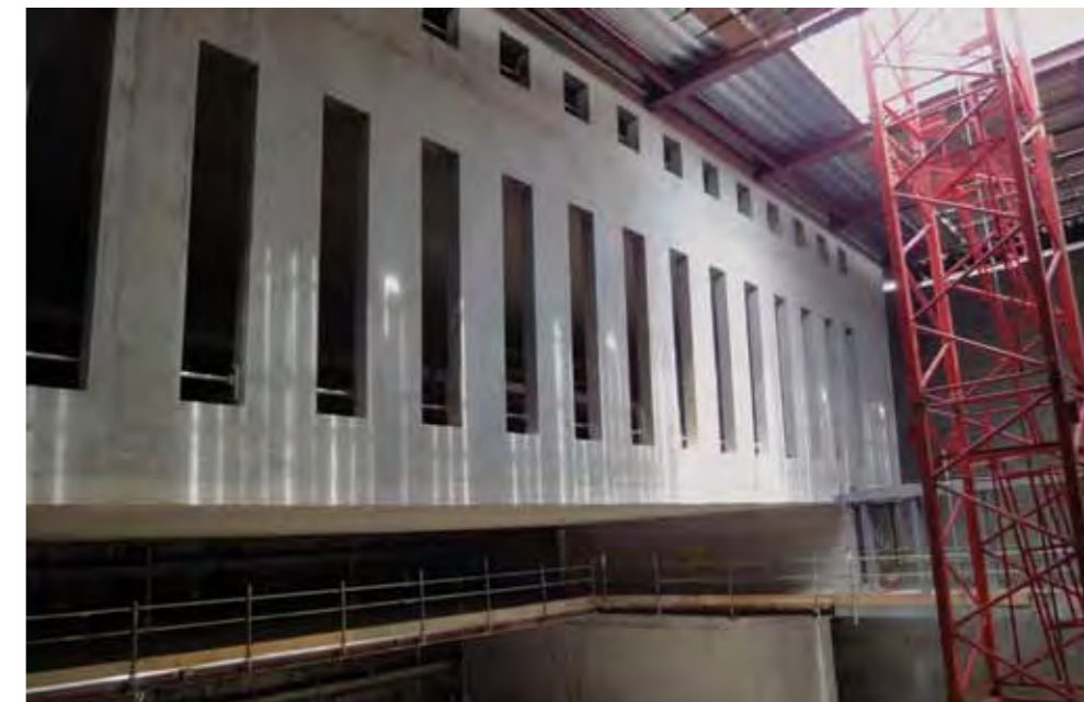
Facing page: artists impression of the finished Blackwell Hall in the Weston Library Above: Blackwell Hall under construction
